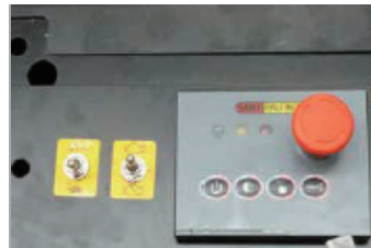
Overload Protection System
