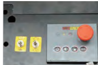
Overload Protection System
